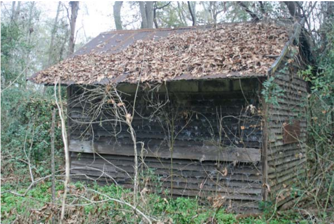
The only other original cabin. This cabin has been moved across the access road. This photo shows the air vents under the overhang.
